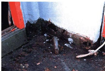
Photograph 1 Corroded accommodation house side structure
